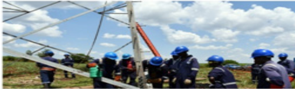
UETCL engineers disassemble a vandalised tower line inside Kakira Sugar Plantation in Jinja District on October 31, 2022. PHOTO/TOBBIAS JOLLY OWINY
